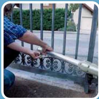
Manual unlocking system to operate the gate in the event of an electrical power cut.
